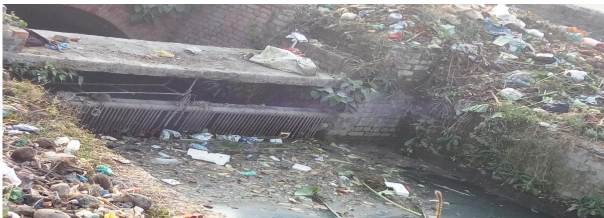
Figure 4: Garbage dumped in the distributary
