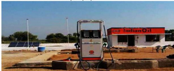
Ground mounted solar installation for petrol pumps
