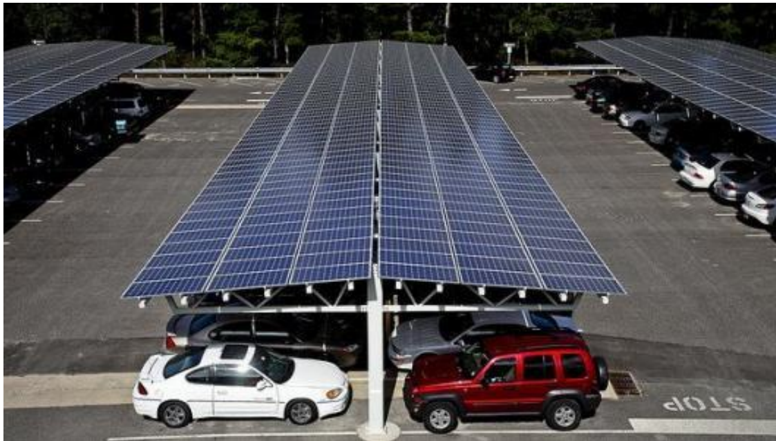
Fig.(3)Electricity generation by solar (By placing solar panels on roof of parking )
