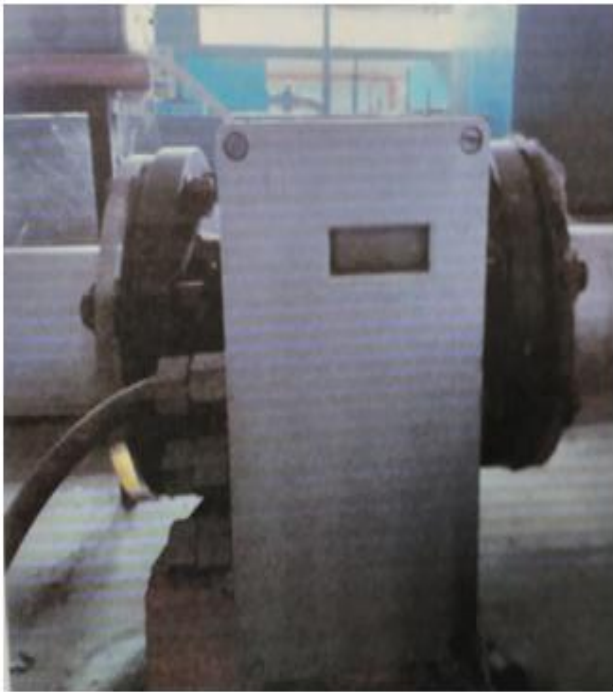
Fig.5. Electro-magneto Meter for Discharge Measurement
