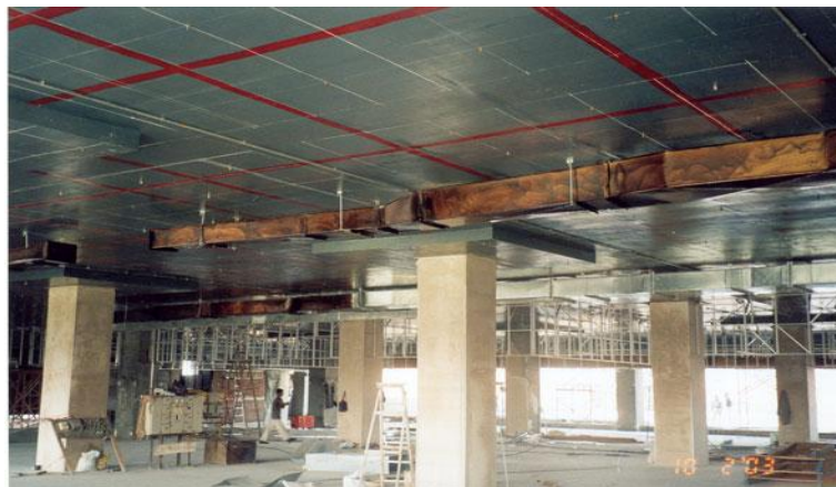
Fig.3 Flexibility in providing AC ducts
