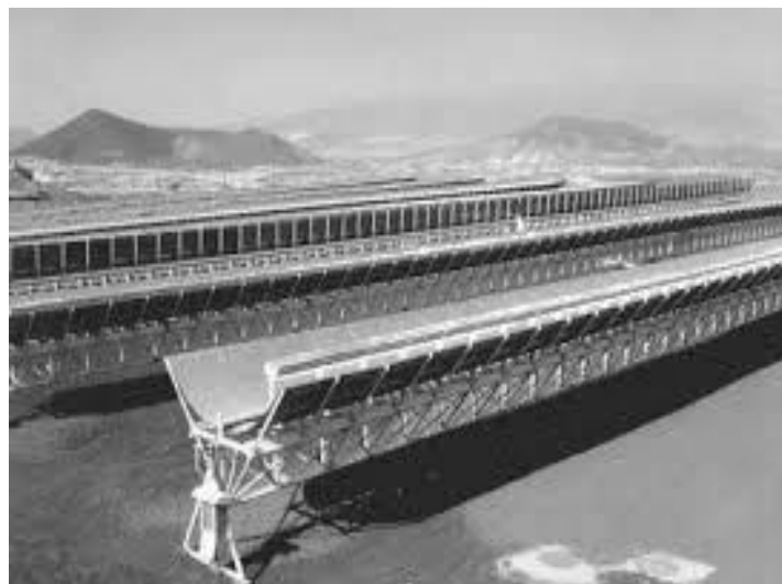
Figure.5: line Focus Parabolic Reflective Trough Concentrator
